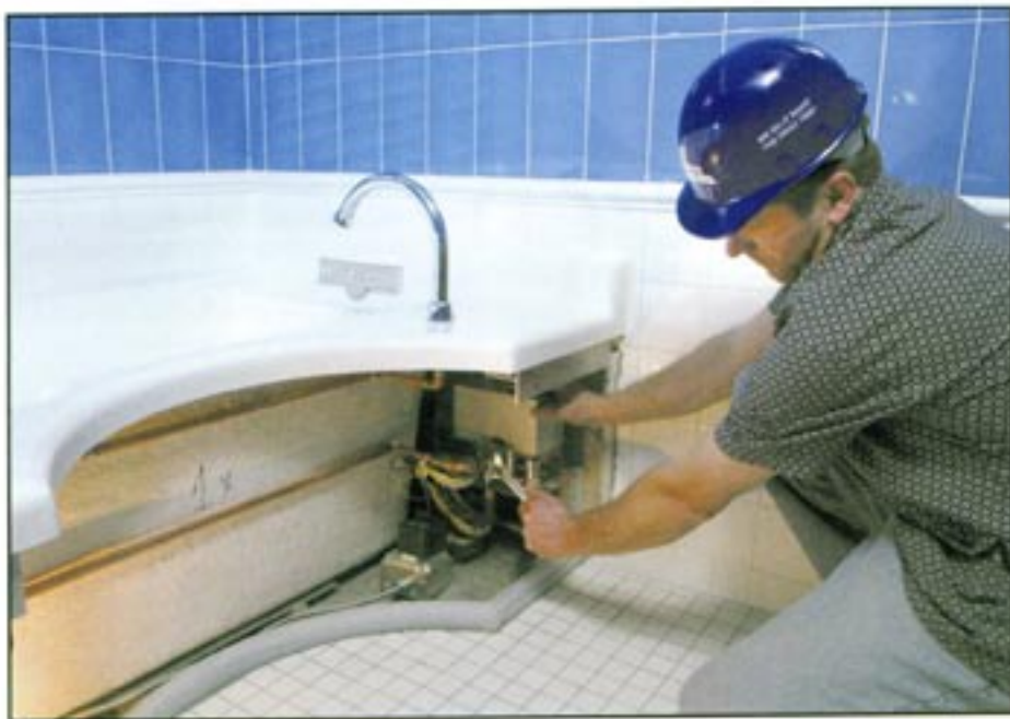
Custom-designed TAG Tubs were installed at the Broadmoor, with minimal effect on existing tile surfaces.
