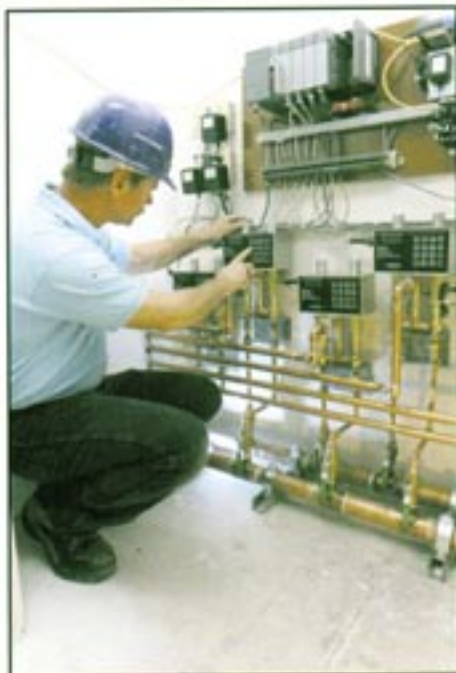
The mechanical closet features six valves that deliver water equally to each showerhead zone.
